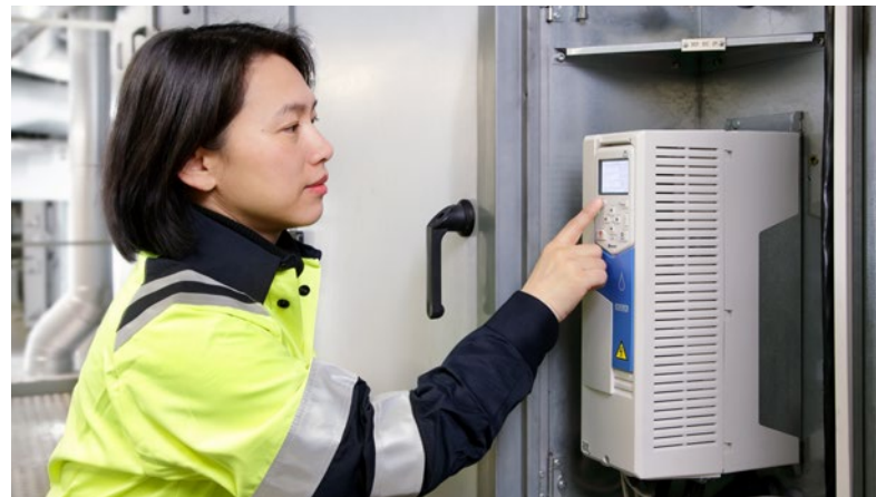
Connectivity panel installation for ACQ580 variable speed drives/variable frequency drives (VSDs/VFDs).
